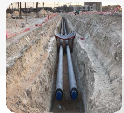
COOLING CHILLER PIPE
