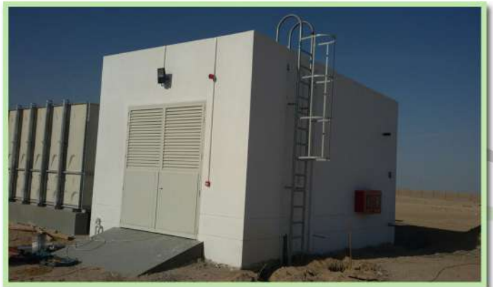
Pump Room With GRP Water Tank And Water Treatment Plant
